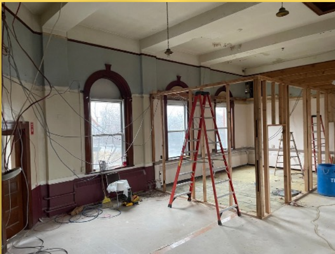
Arched windows that will need restoration.
